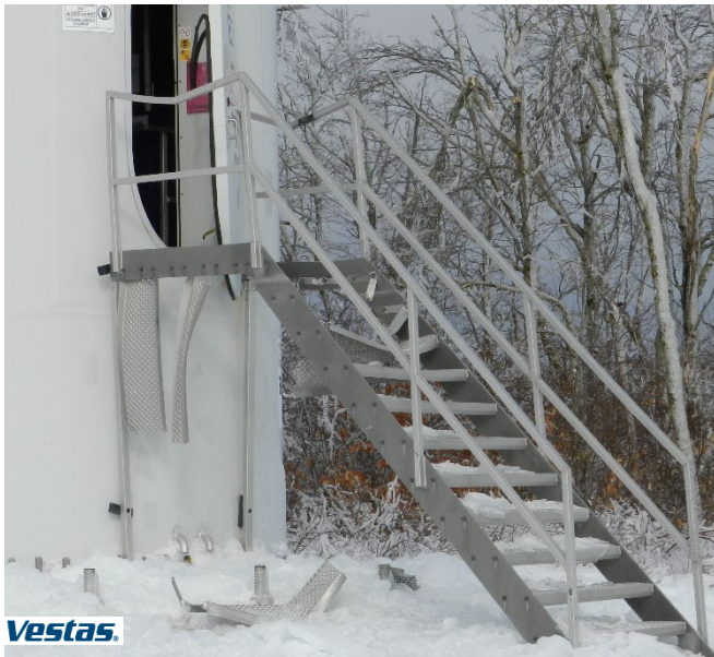
Figure 19: Damaged stairs from an ice fall
